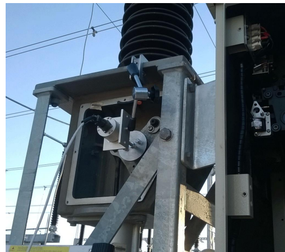
Figure 2: Digital rotary transducer mounted on ABB LTB 245 kV SF6 circuit breaker
