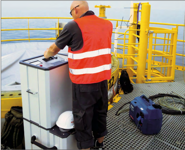
TDS 60 in operation on the "Baltic 1" wind park (Baltic sea).
